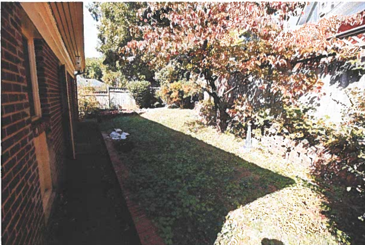
Back East Corner of the property looking to the high point of the lot – The property rises up in back yard. The existing retaining walls need to be replaced
